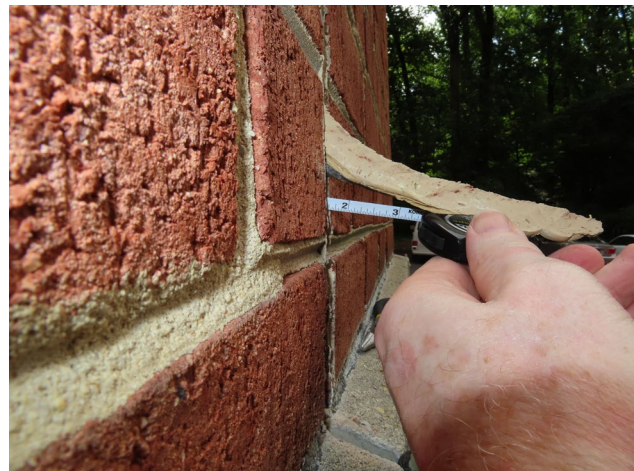
1998 Resto, Superficial Expansion Joints 2" into 4" Brick
